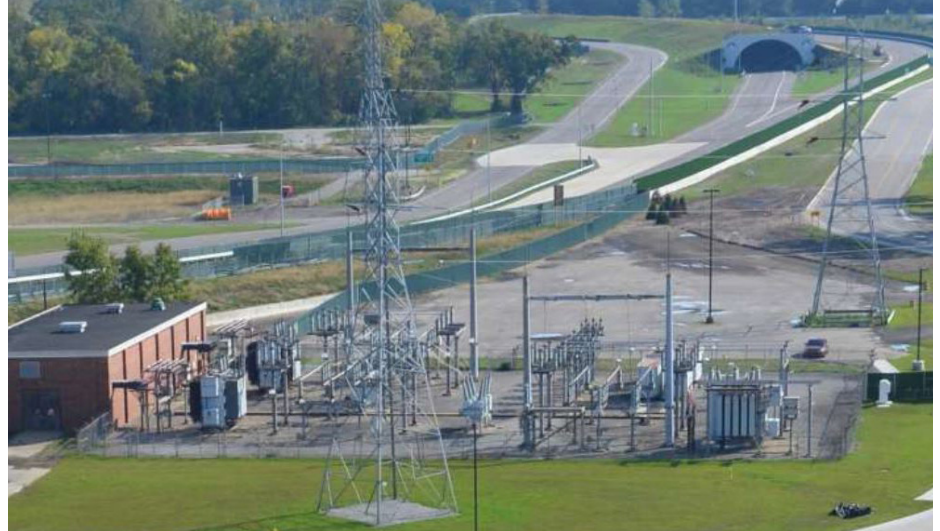
Existing electrical infrastructure includes a 90MW substation with 2.2MW off-grid backup
